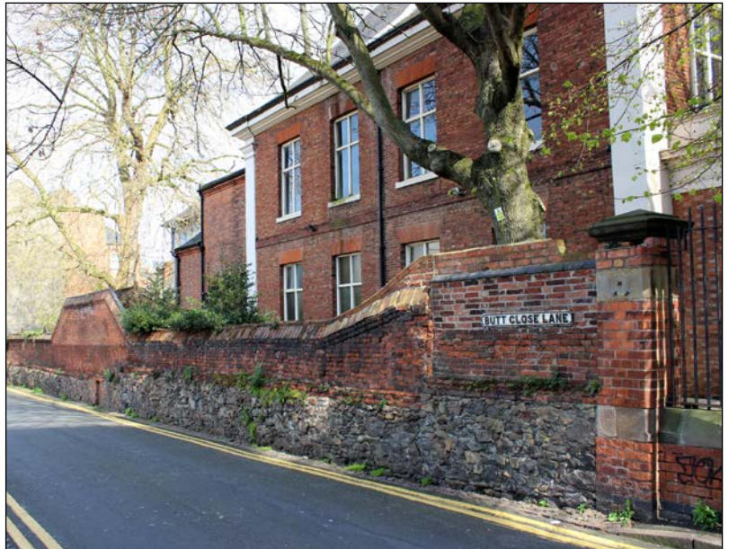
The boundary wall on Butt Close Lane is made of a of stones and bricks of varied styles and likely dates from the 18th Century.
