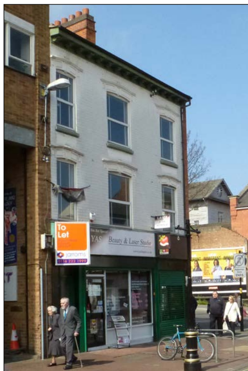
Inappropriate replacement windows which have 'flattened' out the façade.
