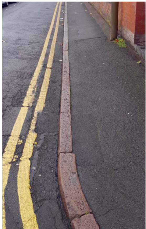
This Mountsorrel Granite Kerb on Blake Street – provides a strong and characterful edge to the pavement.
