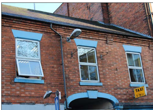
Inappropriate windows at 79 Church Gate.
