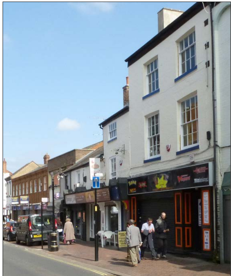
The restoration of traditional windows to the upper floors of 39-45 Church Gate has helped restore lost character and contributes greatly to the overall character of the area.
